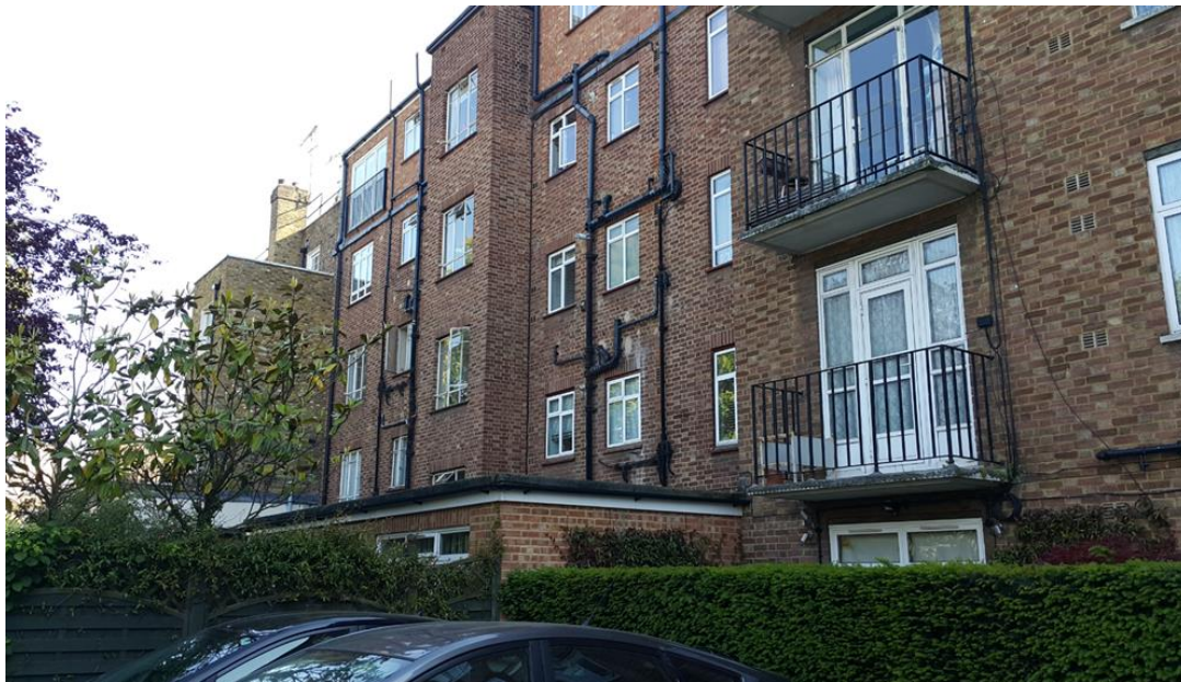
Rear Elevation of Northwick Terrace and the existing flat roof as viewed from the first floor rear window of 13 Northwick Close (top) and existing flat roof as seen from the car park to the rear of Northwick Terrace (bottom).
